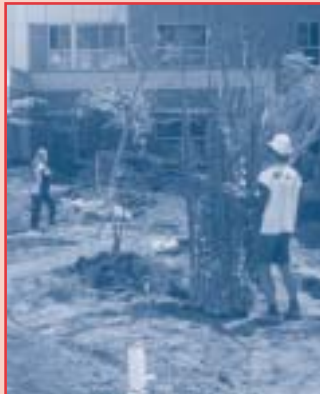
Trees and soil were transported over the walls of JHH and into the garden courtyard via crane
